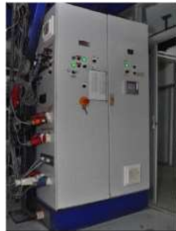
Central Control Cabinet
